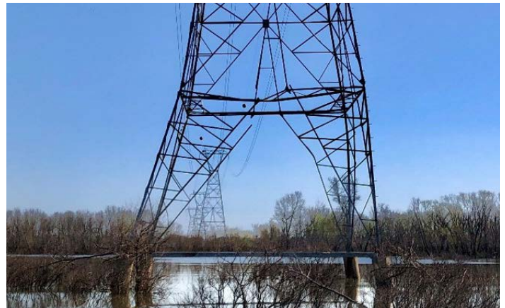
With Bentley's iTwin and Power Line Systems applications, they created a digital twin and saved four to six weeks designing a stabilization solution.
